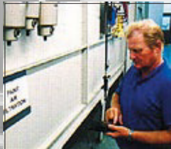
Compressed Air Analysis
